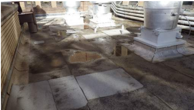
1968 worn membrane / ponding (Building 6, area Z)
