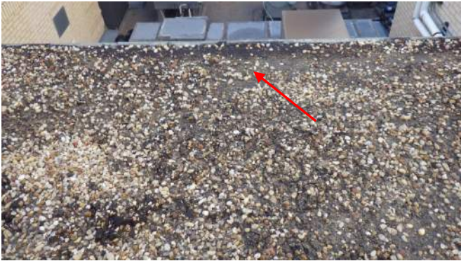
1968 worn / cracking membrane (Building 6, area S)
