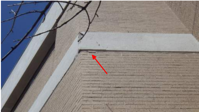
Trauma Center cracking brick at precast
