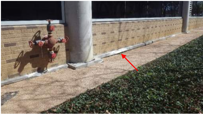
Pavilion damaged flashing
