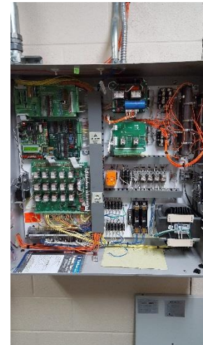
8. Typical of Motion Control Engineering (MCE) Controls Installed as an Upgrade in 1996, '99 and 2000 on Units #3, 4, 5, 6, 7, 26 & 27
