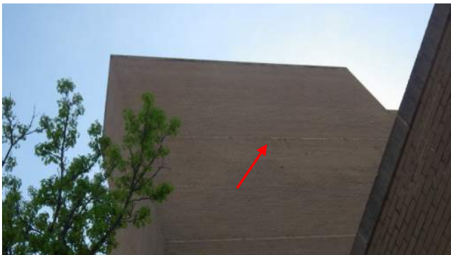
1972 deteriorating brick joints
