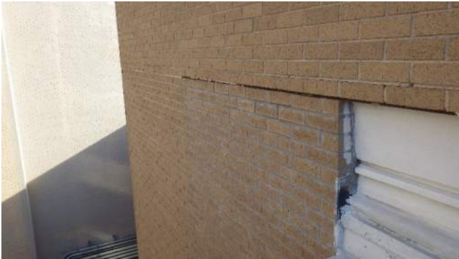
1972 deteriorating brick joints
