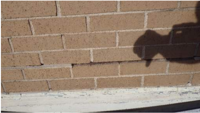
1972 deteriorating brick joints
