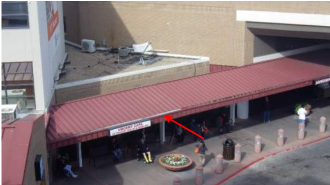
Trauma Center damaged canopy
