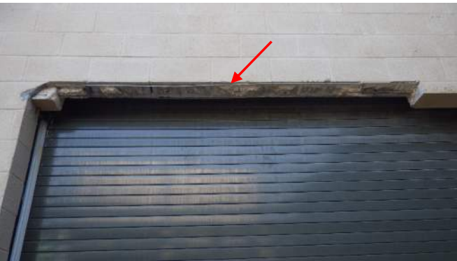
Pavilion Parking Structure damaged door lintel
