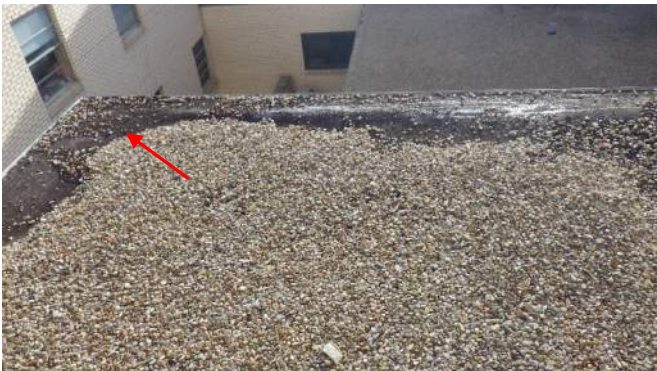
1968 gravel erosion / worn membrane (Building 6, area S)
