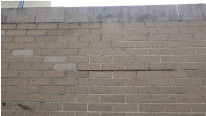
1972 deteriorating brick joints
