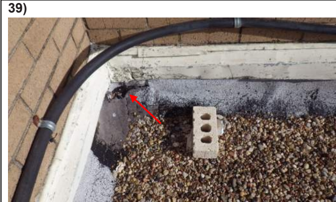
1972 parapet flashing damage
