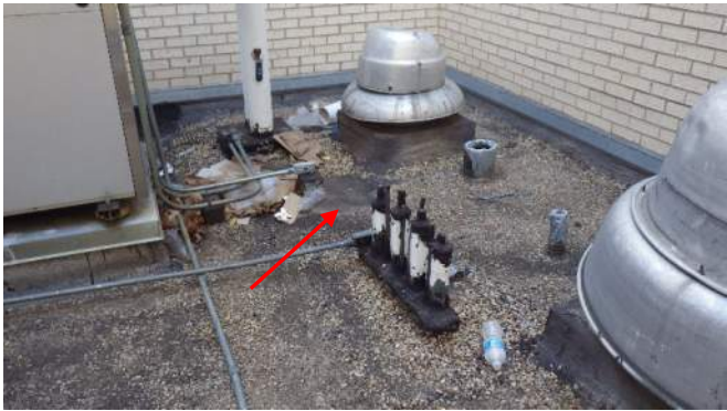
1968 gravel erosion / worn membrane (Building 6, area R)
