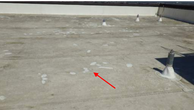
Pavilion roof hail damage
