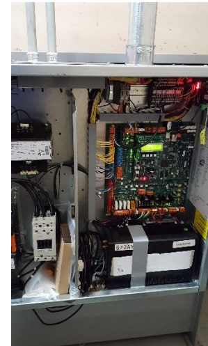
12. Typical of ThyssenKrupp TAC 32H Controls on Units #1-2 at the 1350 JPOC Building Upgraded in 2016
