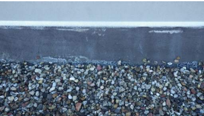
Trinity Springs flashing
