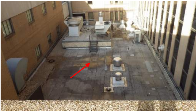
1968 worn membrane / ponding (Building 6, area Z)
