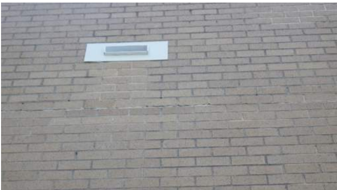
1972 deteriorating brick joints
