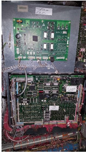
9. Typical Otis Gen2 Controls on Units #32, 33 & 36-41 located in the Pavilion Building installed in 2007
