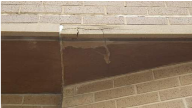
1972 deteriorating brick joints
