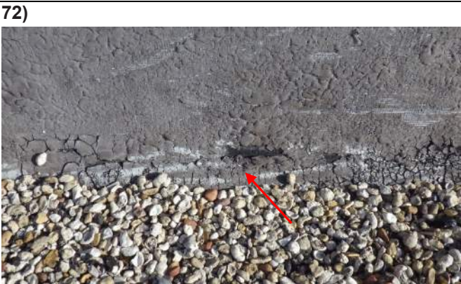
Entry Building flashing deterioration
