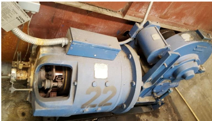
7. Typical of Dover 105 Geared Hoistmachine with Low Support Found on Units # 22 & 23
