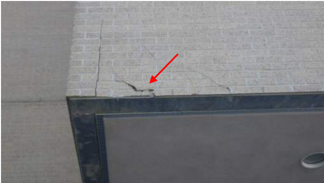
Pavilion damaged soffit at dock
