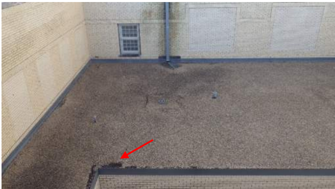
1968 gravel erosion (Building 6, area T)
