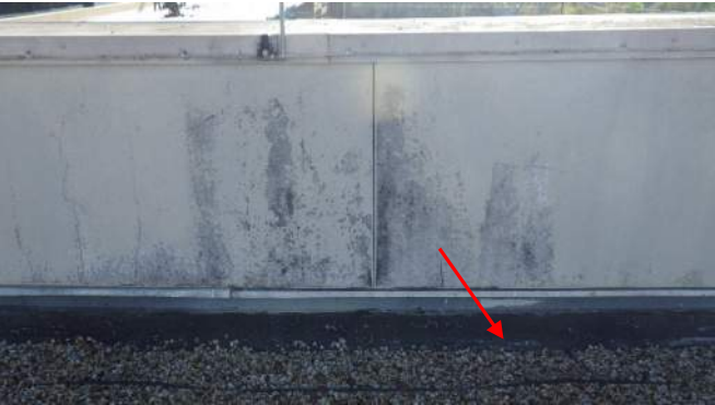
Trauma Center deteriorated flashing
