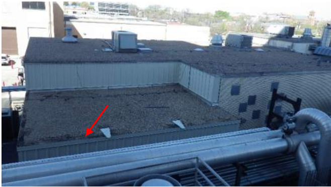
1968 Plant - gravel erosion
