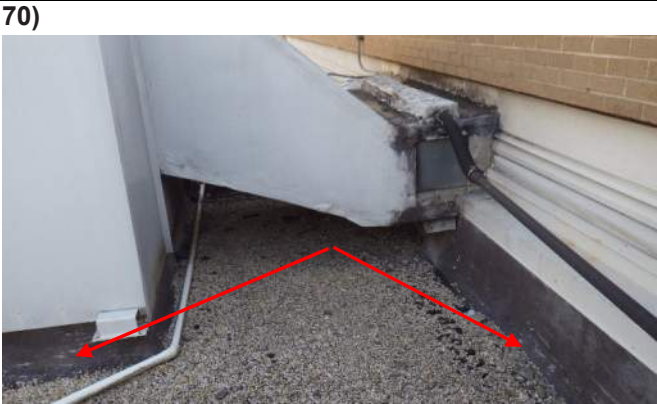
Entry Building flashing deterioration
