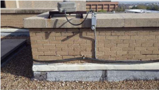
1972 deteriorating brick joints
