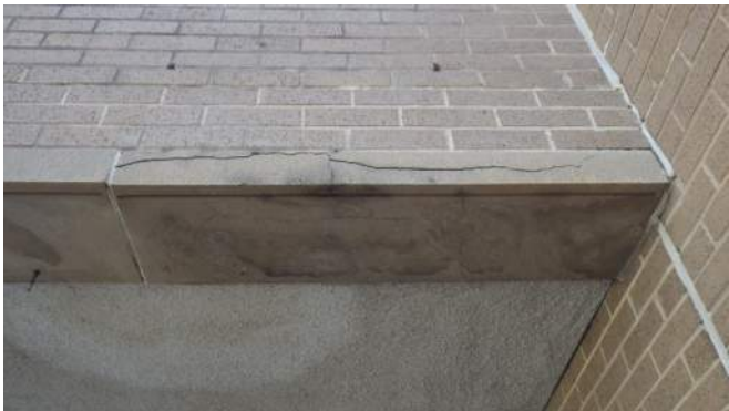
1972 deteriorating brick joints
