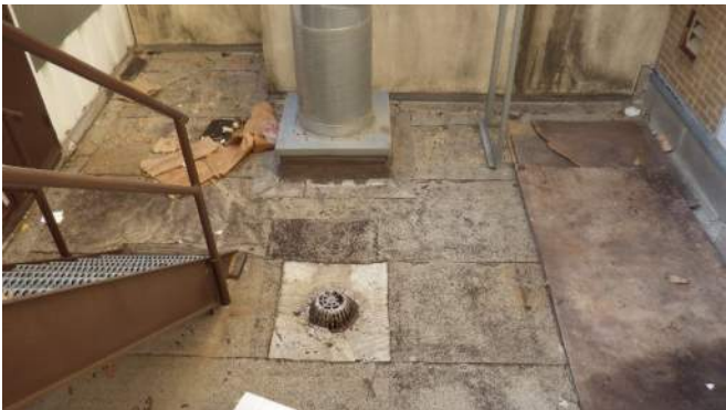
1968 worn membrane / ponding (Building 6, area Z)
