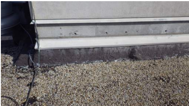
OPC roof flashing
