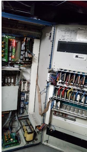
1. Typical of Obsolete Controls for Units #29, 30 & 31. Montgomery Ultron Mirpoms Installed in 1993
