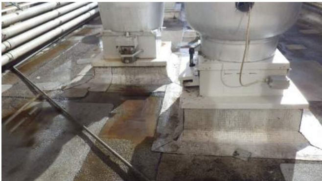
1968 worn membrane / ponding (Building 6, area Z)
