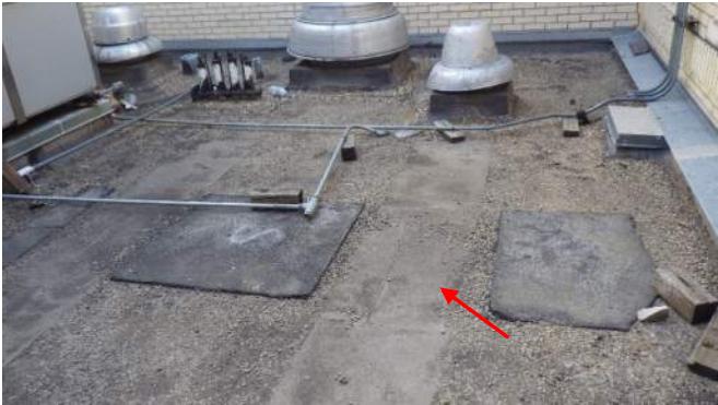
1968 gravel erosion / worn membrane (Building 6, area R)
