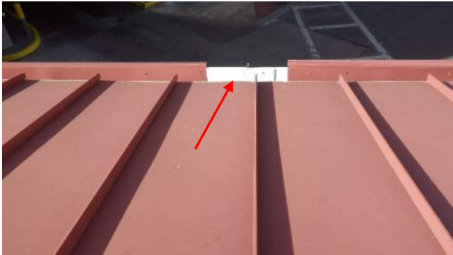
Trauma Center damaged canopy
