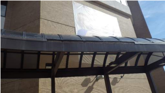
Entry Building canopy damage
