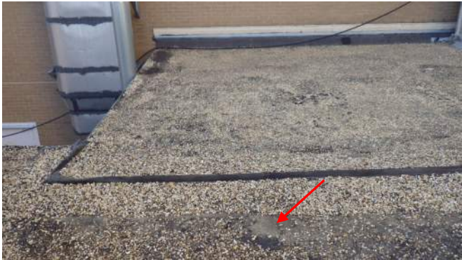
1968 gravel erosion / worn membrane (Building 6, area S)
