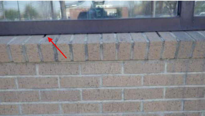
Plant window sill deterioration
