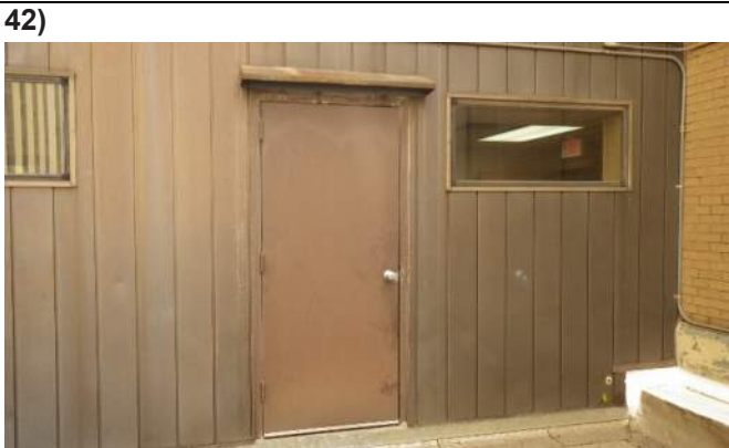
1972 metal panel condition
