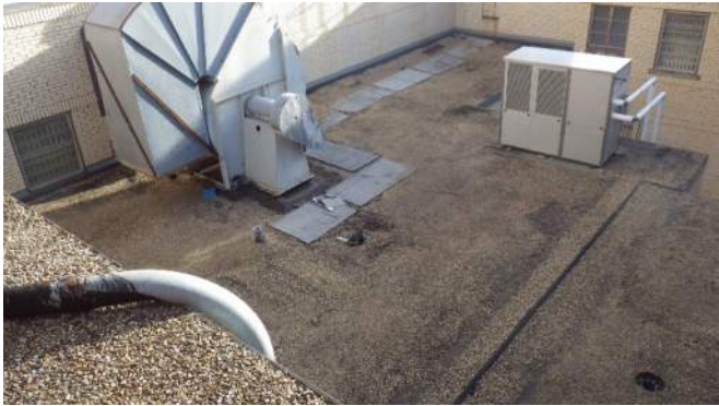
1968 worn membrane (Building 6, area S)
