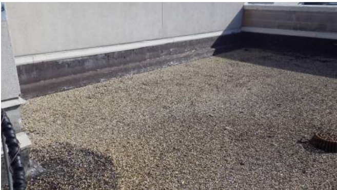
OPC roof flashing
