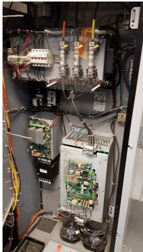
11. Typical of ThyssenKrupp TAC 50 Controls on Units #1-3 at the 1400 JPOC Building Upgraded in 2010
