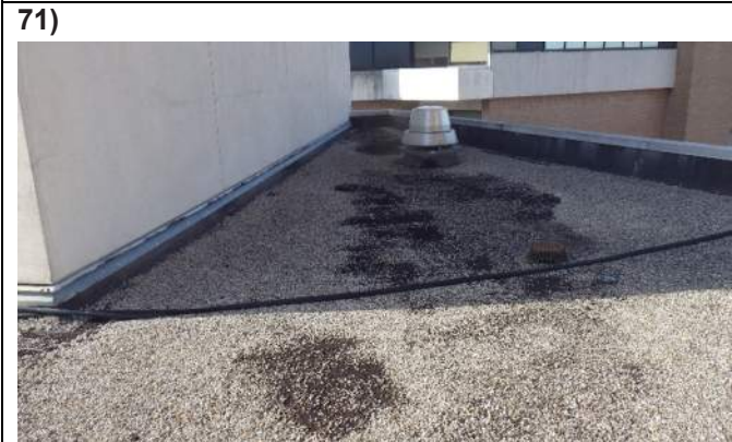
Entry Building roof gravel erosion
