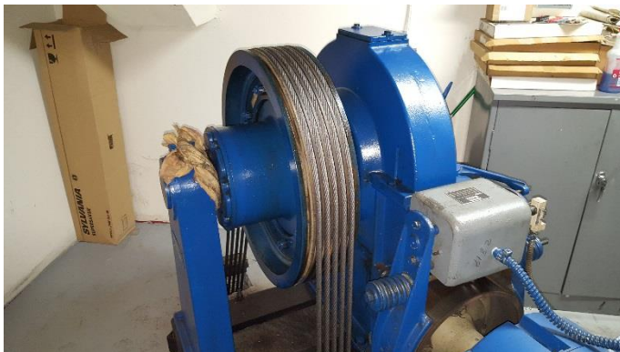
3. Typical Montgomery 208 Hoistmachine with Low Support and Limited Lifespan. Found on Units #12, 13, 14, 15, 20, 21, 29, 30 & 30
