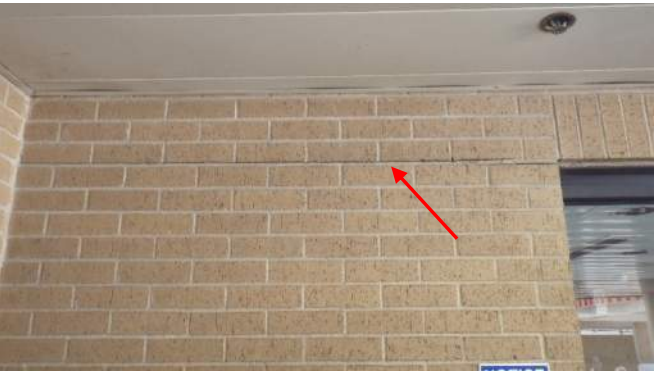
Trauma Center loose brick joint
