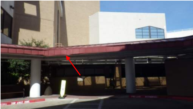
Trauma Center damaged canopy
