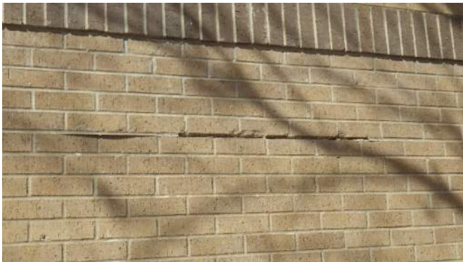
Tunnel brick joint deteriorating
