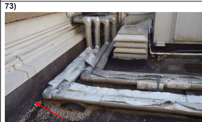
Entry Building flashing deterioration
