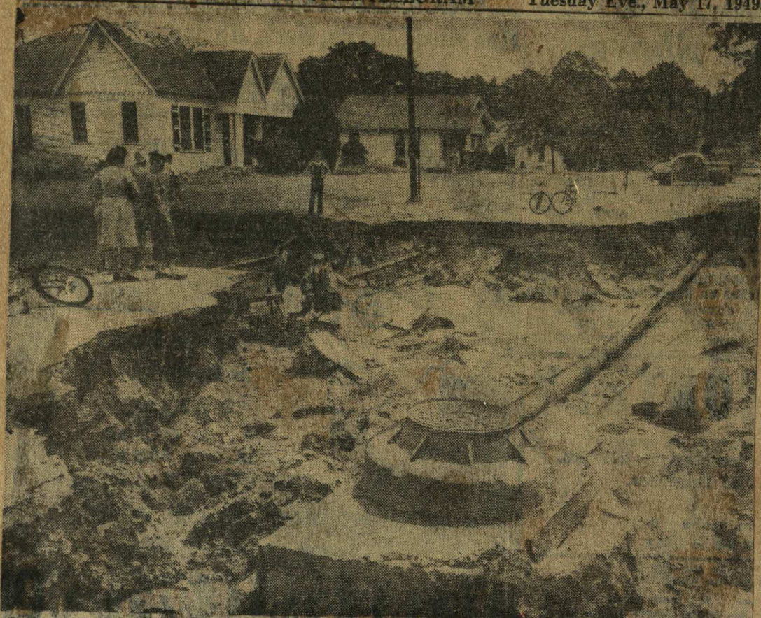
NATURE'S SCOOP —A culvert at the 3700 block of Yucca was washed away and added this scene to the picture of flood damage in Fort Worth Tuesday. —Star-Telegram Staff Photo.
