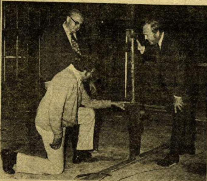
Standing from left to right is Pat McCoy and Commissioner Richard T. Anderson, inspecting part of the plumbing installation at the new sub-courthouse is Dick Powell.
